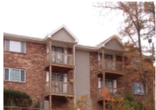
The Crescent Hills Apartment Complex renovated by the Community Alliance of Metropolitan Parkway won AHAND's 2005 Project of the Year award.
